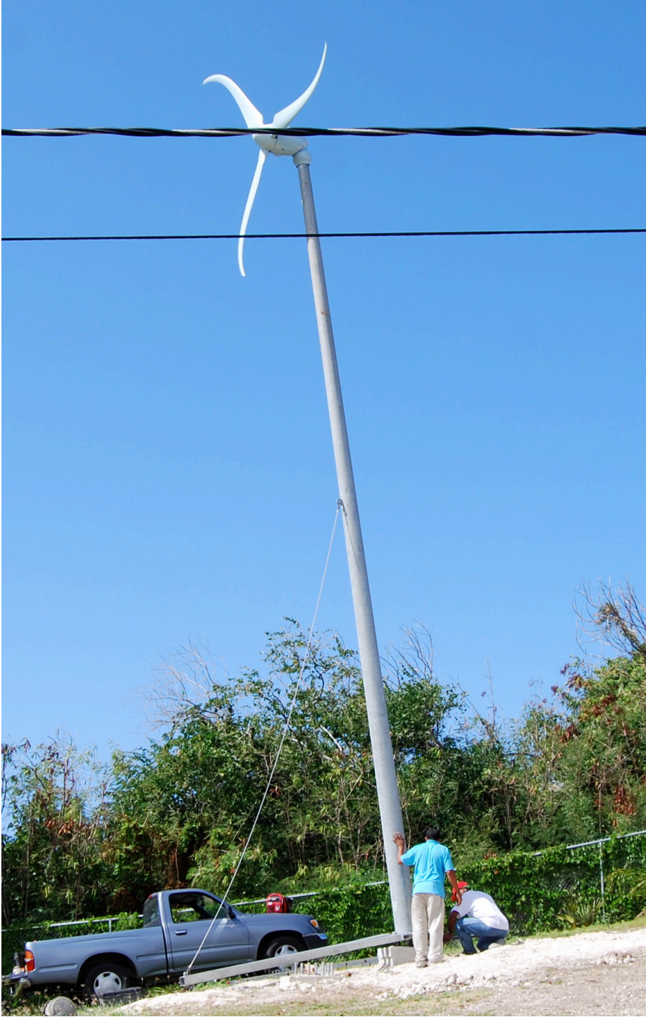
The wind turbine
